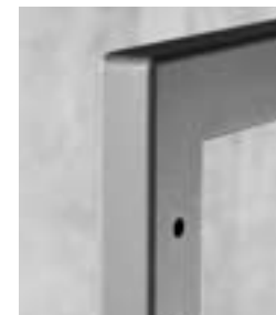
Upper corner shows no weld
